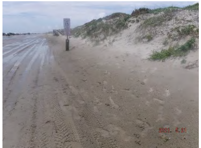
Picture 106: UD14JLM Bearing: West Date: 5/21/2021
